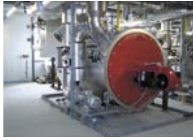
Boiler with extracted hot air exchange system
